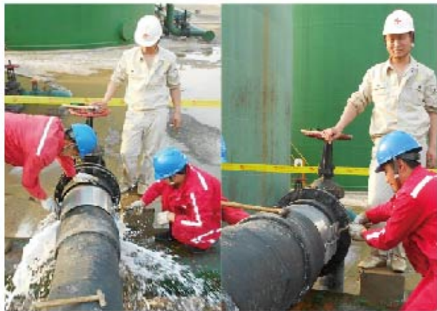
Within 3 minutes, under pressure leakage repairing has done successfully on the DN450 water supply pipeline in Puyang Oilfield.
