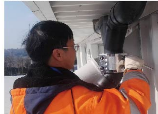
The welding joints of the siphon drainage pipeline break off. For secondary production, they adopt Zhuhong Repair Clamp.
