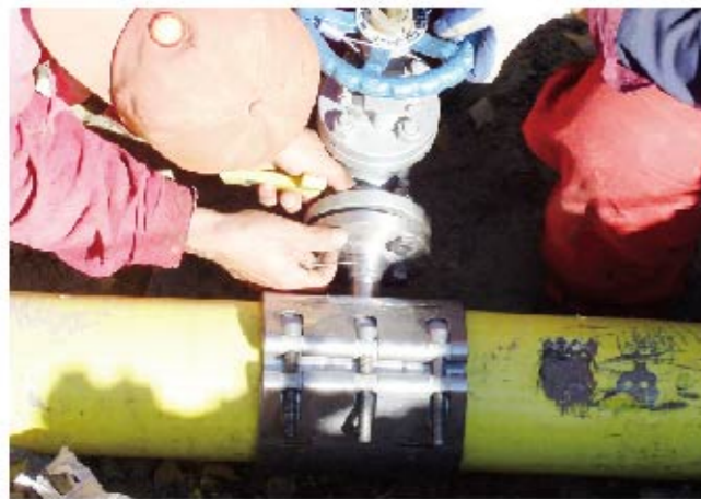
For DN150 pipe with DN20 branch, Daqing Oilfield adopts Zhuhong Multi-Function Tee Clamp to install with hoing and sealing on nonstop pressured pipeline.
