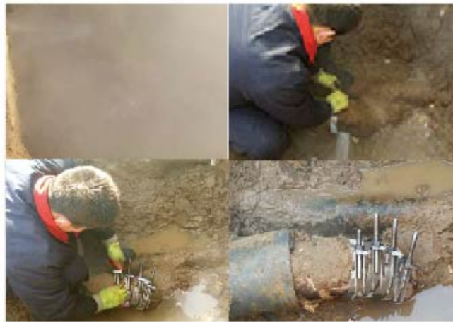
Within 10 minutes, Zhuhong Elbow Repair Clamps have been used to repair the 90° degree elbow of DN150 steel pipe.
