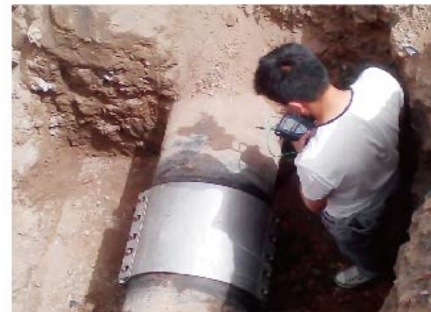
To solve the leakage of DN400 gas pipeline in Shanxi Huarun Gas Company, Zhuhong RCD Double-Section Repair Clamp performs quite excellent in fast repairing.
