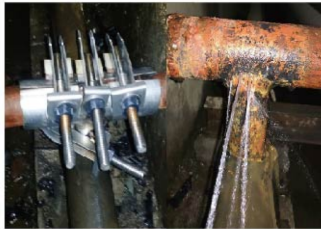
Zhuhong Tee Clamp functions very well on the tee part of DN40 pipelines in the High Railway Station.
