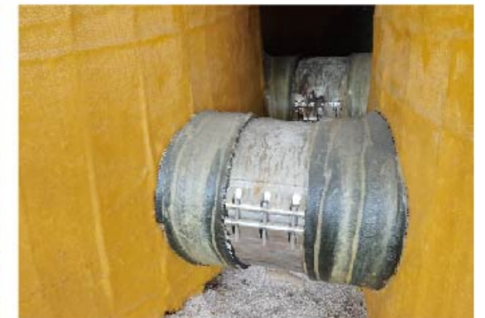
RCD Double-Section also works smoothly to stop leaking between the gap of two oil tanks in Shengling Oilfield.
