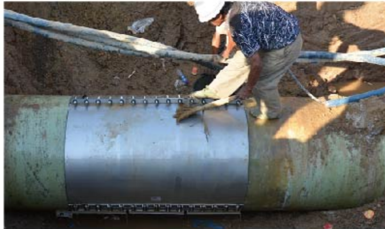
To repair the DN1200 GRP pipe of Hunnan Water Corporation conventionally, they'll have to stop the water pipe for more than 36 hours. However, using the Repair Clamp of Zhuhong instead just make it within 2 hours.
